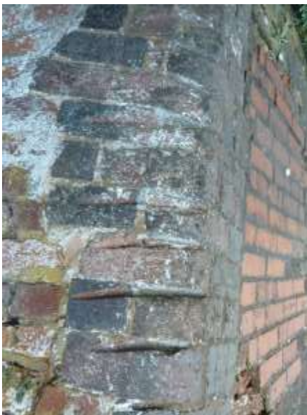
Rope marks on a bridge wall
